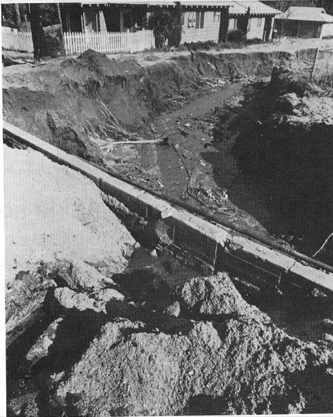
Water eroded the ground at Grand and Adelpa in the City of Lake Elsinore.
